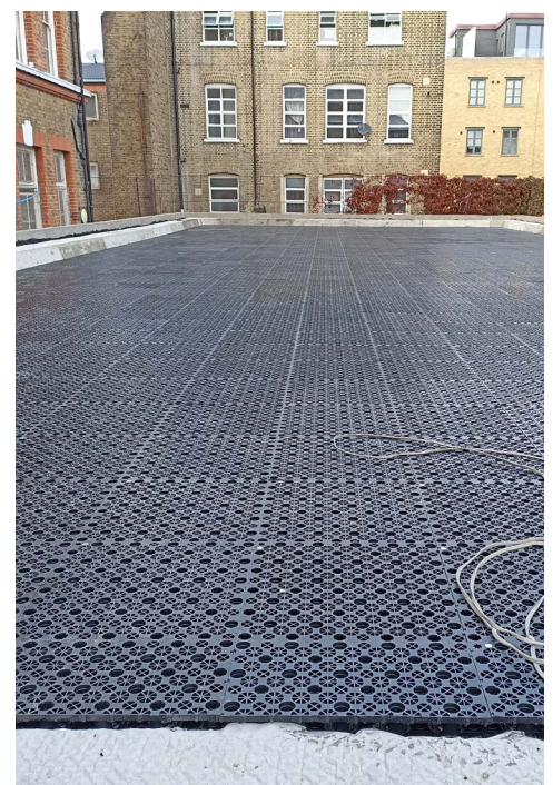
Figure 1. Example of RoofBlox Blue Roof on a School in London. © Aco Building Drainage
