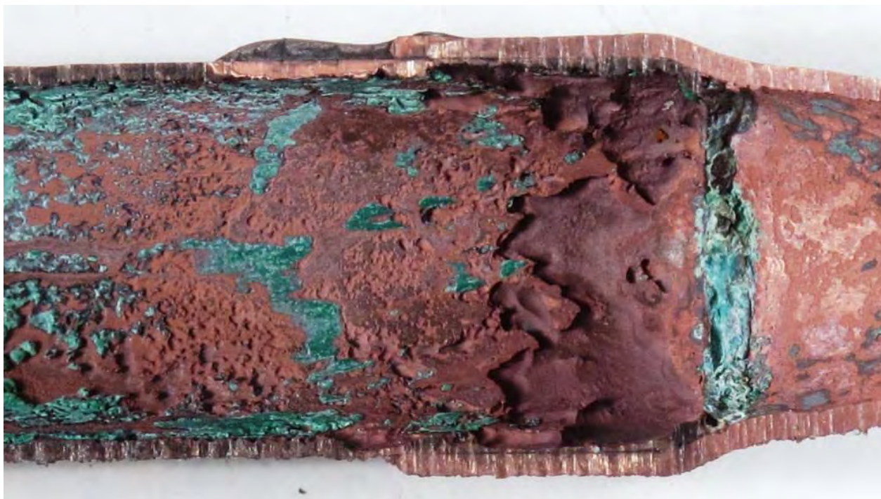
Figure 3 Erosion corrosion on hot water recirculating return pipe © P Munn
