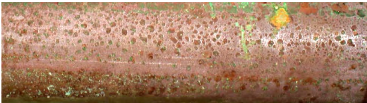
Figure 12 Appearance of formicary corrosion on the outside of copper pipe after removal of lagging © P Munn
