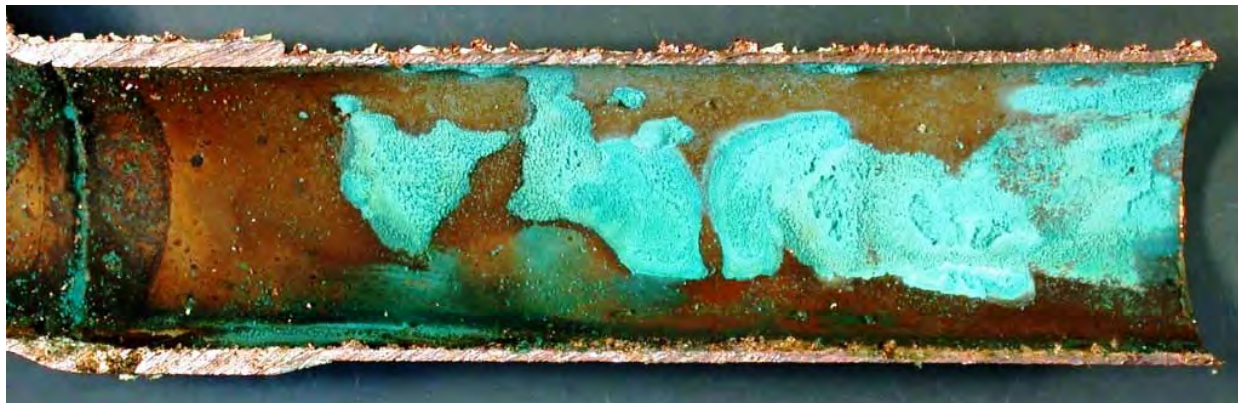
Figure 2 Build up of an unstable, irregular carbonate layer on the pipe bore, resulting in blue water © P Munn
