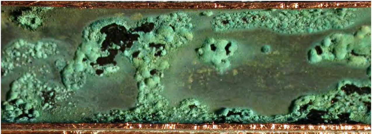
Figure 8 Microbial Influenced Corrosion on a cold water pipe © P Munn
