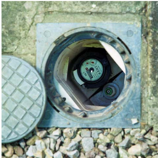
Water meter. ©Sheila Terry/Science Photo Library
