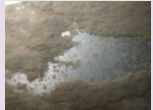
Bio-film after System Flushing
